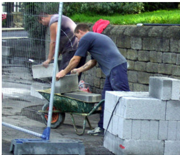
The construction of the small stone walled garden is already well under way.
